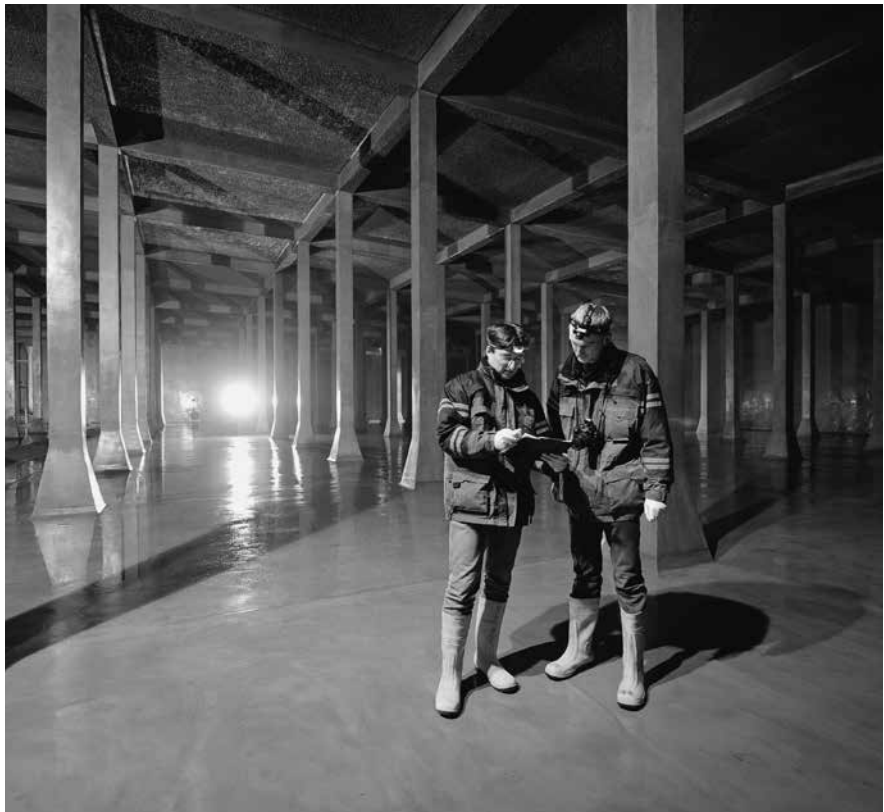
Fig. V-58: Experts from the Research Institute of the Cement Industry in action in drinking water containers – component consultation and testing of the compliance with the requirements pursuant to the technical rules of the DVGW W 270, W 300, W 347.
