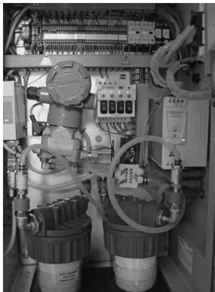
Fig. II-3: Long-term sampler for determining the biogenic CO 2 emission in exhaust gas
