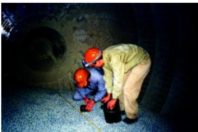
Fig. 3: Mill experiment for the optimisation of energy consumption and the particle size distribution of the cement
